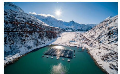
Lac de Toules: Floating solar power system in the Swiss Alps ©Romande Energie
